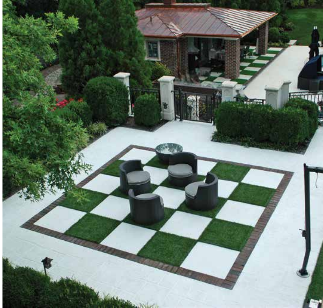
THE SECOND PHASE WAS THE MIDDLE TERRACE WITH TWO CHECKERBOARD SECTIONS. MORE THAN 6,000 SQUARE FEET OF DECORATIVE CONCRETE WAS INSTALLED AT THIS NEW JERSEY PROPERTY.
